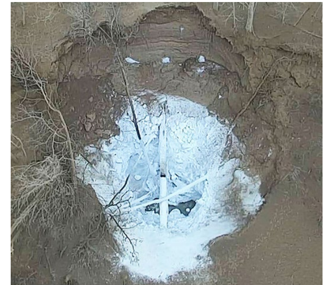
Rupture of a carbon dioxide pipeline near Satartia, MS in February 2020
